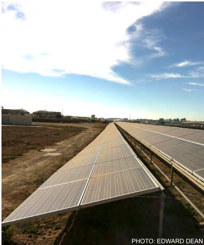
Solar photovoltaic panel ground array (below).
