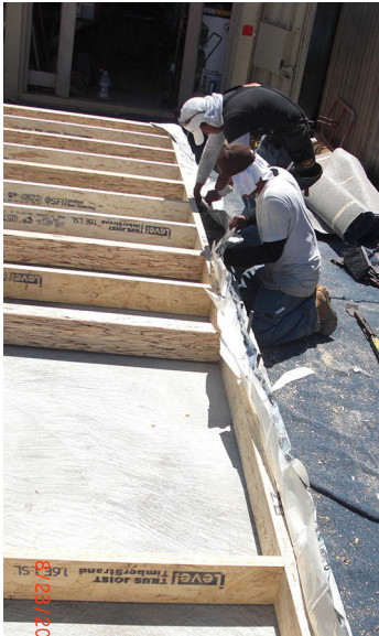
(Above) Airtightness: attaching the gaskets to the bottom of the wall frame. (Photos courtesy of John Steed Homes.)
