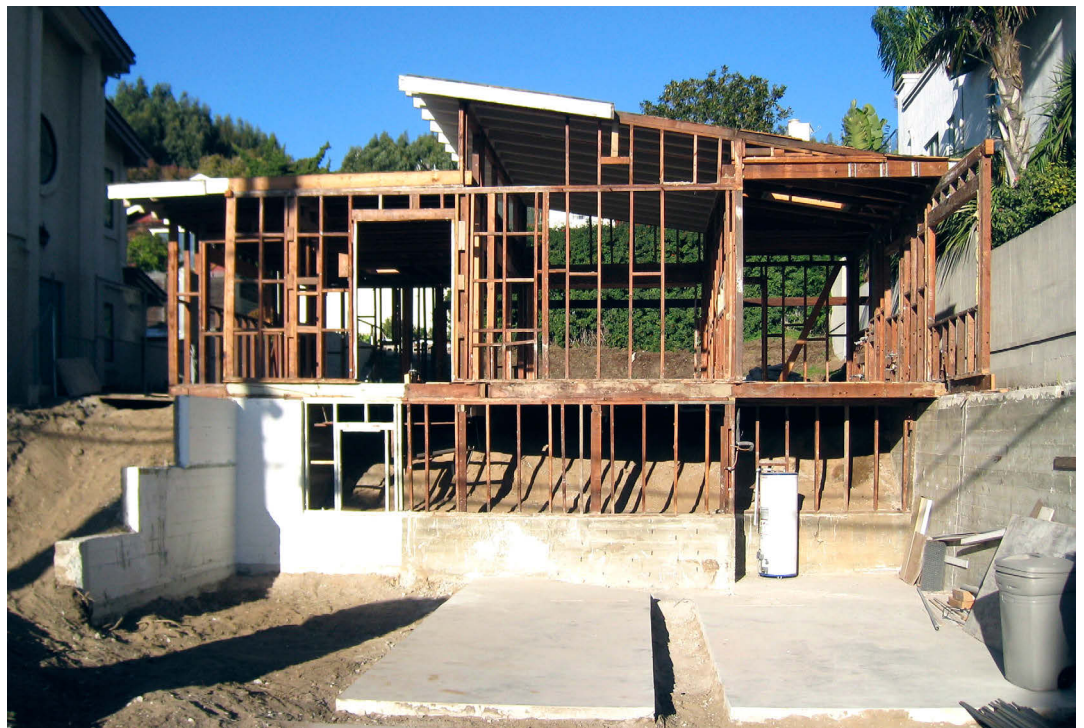
(Right) View of final “deconstructed” original house, with some rough framing and foundations from the rear half of the 1959 house salvaged for the new structure. The west half of the new house would be mostly new construction.
