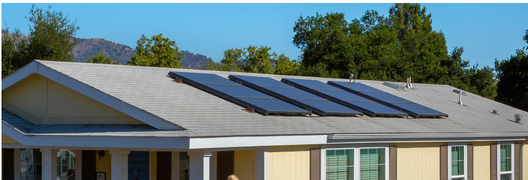
(Left) Initial installations of the solar PV systems on the roofs of the Oak Haven houses.
