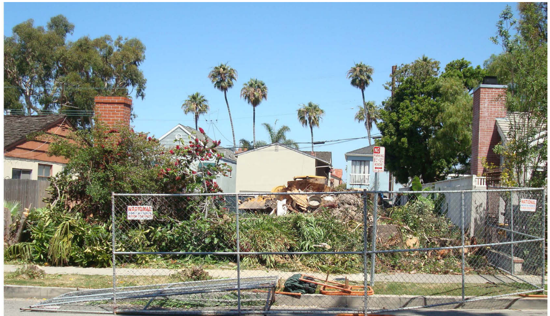
(Above) Original house on the property at 703 Heliotrope torn down for new construction.
